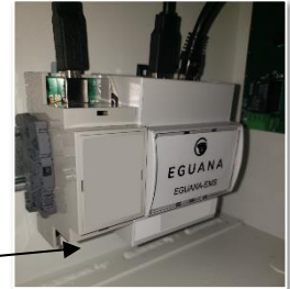
Figure 19: Meter communication connection.
